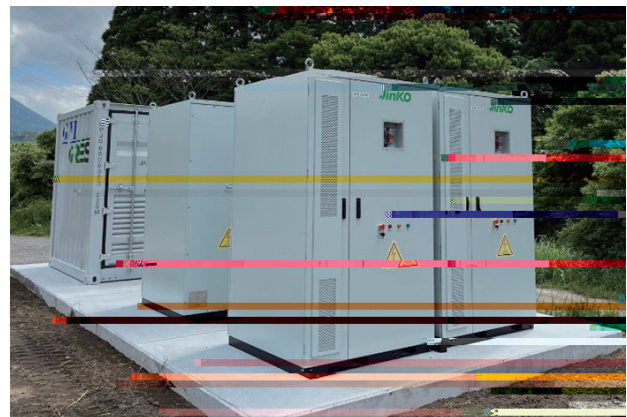
Fig. 2 Jinko ESS 215kWh DC Blocks
